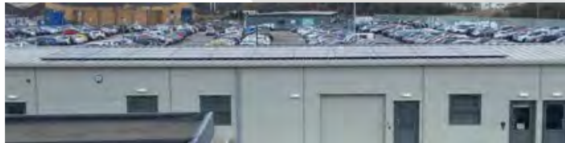
Hull University Teaching Hospitals PV Installation
